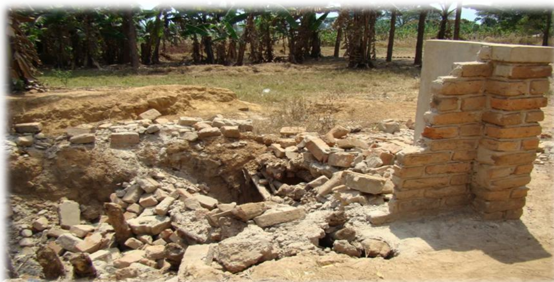
A collapsed toilet built with no value for money at Nyamutukuza village in Kibondo district in Kigoma region. The photographs were taken by during a PETS training conducted by Haki Kazi.
