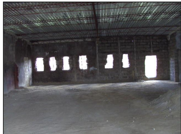
dilapidated structure to be turned into classrooms
