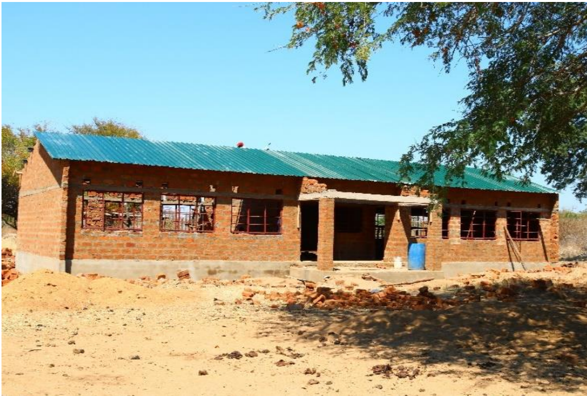
The extension of a 1 x 1 to a 1x2 classroom block. The extension is the right side added.
